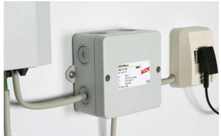
Protection of a telecommunication interface (telephone connection) at the service entry point
