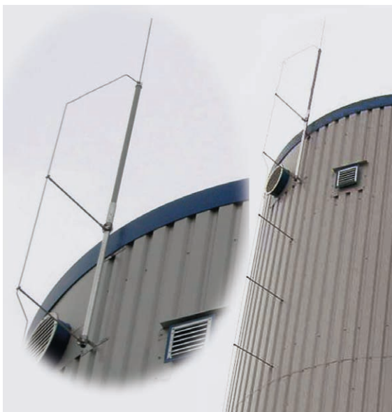
Figure 7 Protection of a fermenter made of metal sheets by means of an isolated air-termination system (source: Büro für Technik, Hösbach)
