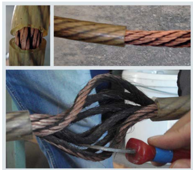
Figure 6 Fault detected by means of the method
