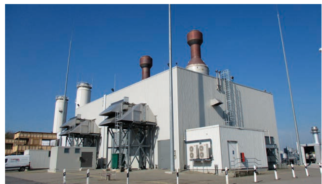
Photos: Isolated external lightning protection system with HVI installation on the Werne compressor station
