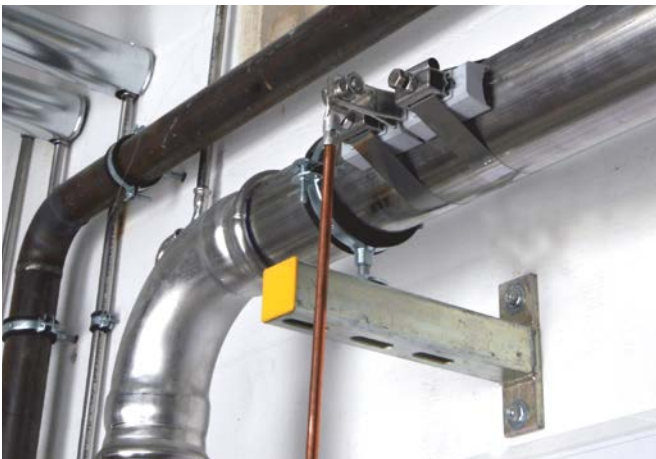
Installed at a StSt pipe.
