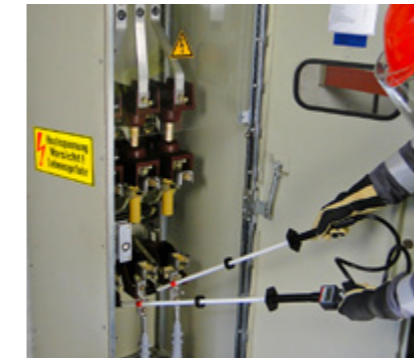
Test with HS 11 at 10 kV transformer
