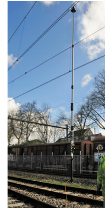
Test at a rail overhead line
