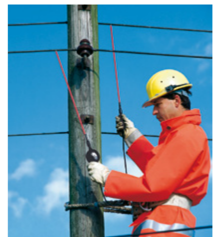
Extensions for higher safety during test at overhead lines and busbars
