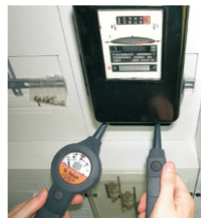
Integrated 350W-load for fast start-up tests at electricity meters
