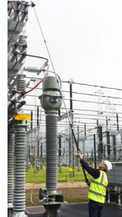
Test at a 36 kV compensation system
