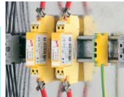
Protection of fire alarm systems
