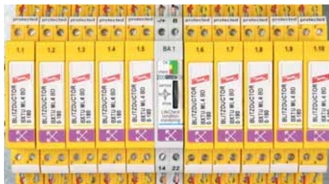
Nainstalovaný DEHRecord Condition Monitoring System.
