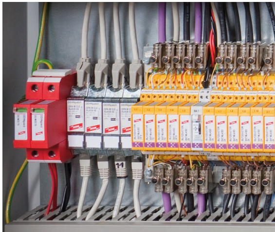
Figure 11 Example of surge protective devices in a pitch system
