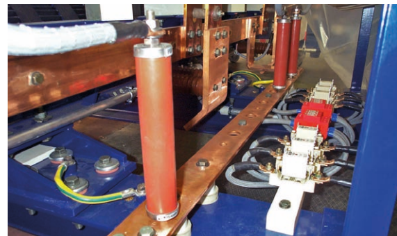
Figure 9 DEHNmid medium-voltage arresters installed in a transformer for wind turbines
