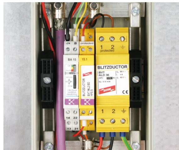
Figure 10 Protection of wind measurement equipment (anemometer)
