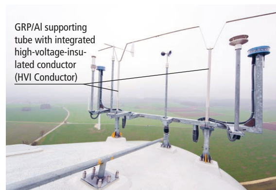
Figure 2 Example of an air-termination system for the weather station and the aircraft warning light
