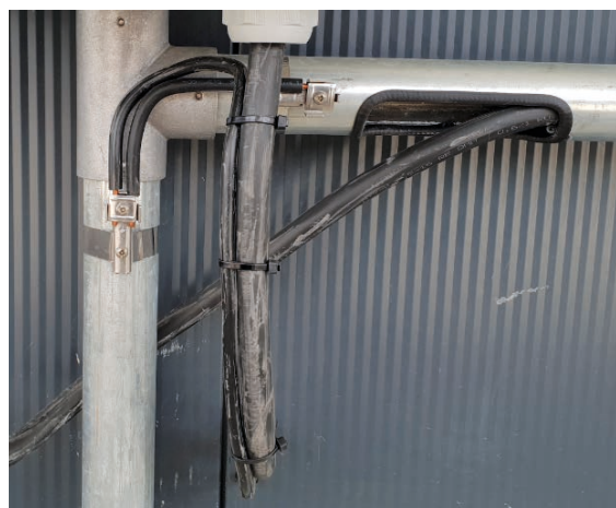
Figure 5 Equipotential bonding of metallic structural components by means of pipe clamps tested with lightning currents
