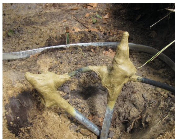
Figure 1 Anti-corrosion tape fitted in a form-fitting manner around the clamp connection in the soil
